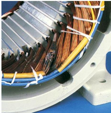
Figure 10: Failure of stator winding, EASA
