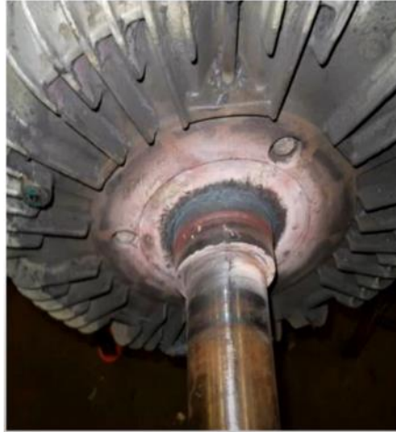
Figure 3: Shaft brown/blue discoloration is a sign of excessive heat damage
